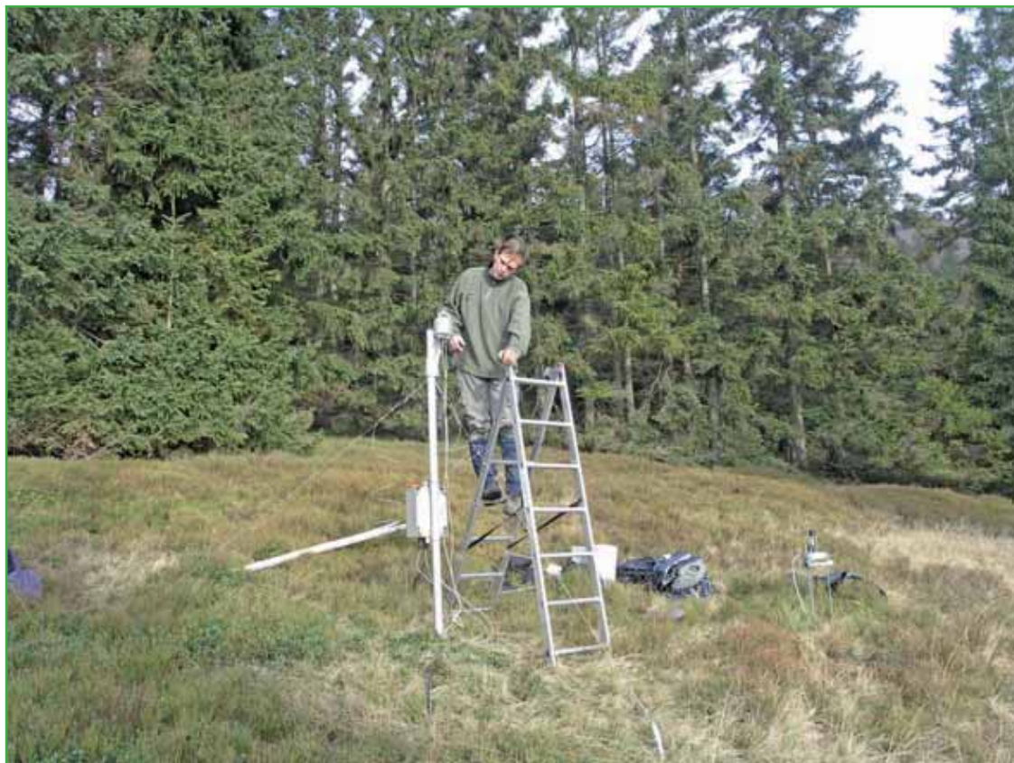
Obr. 4.2.1.11: Instalace meteostaničky Installing meteostation
